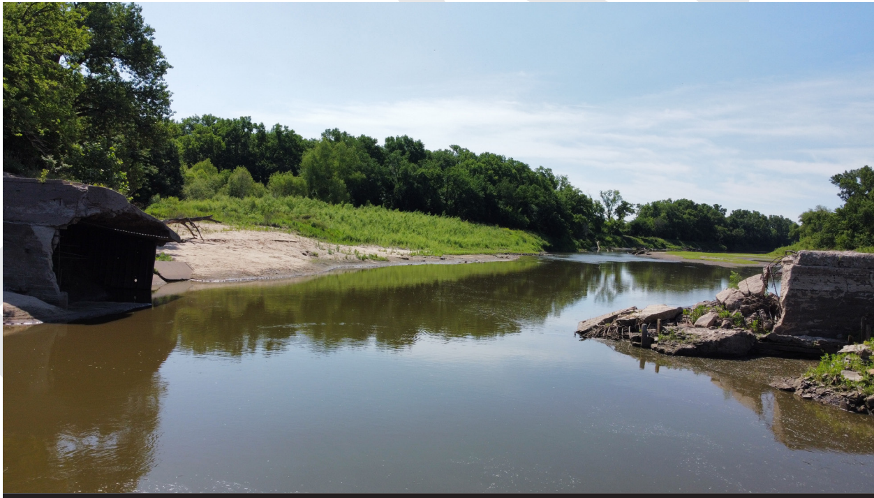
Figure 3. Marysville Dam breach (looking south)
