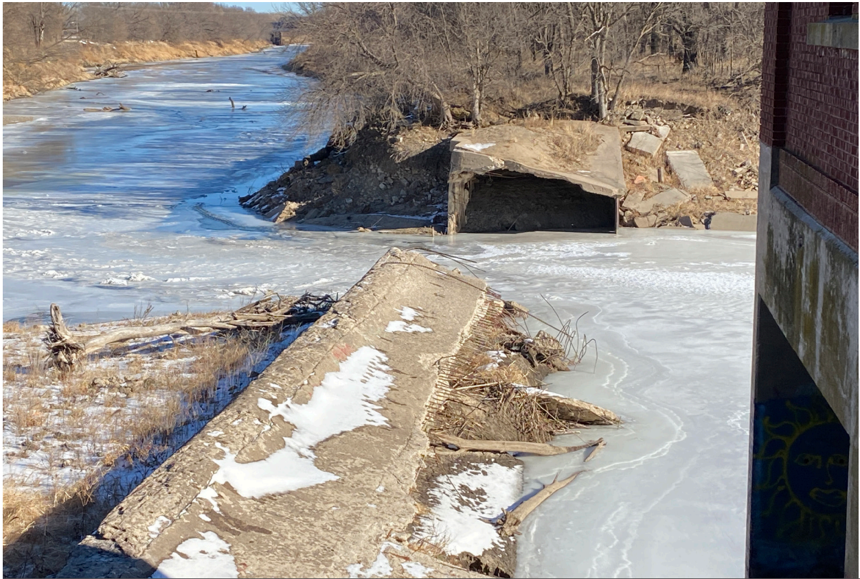
Figure 2. Marysville Dam breach (looking northeast)
